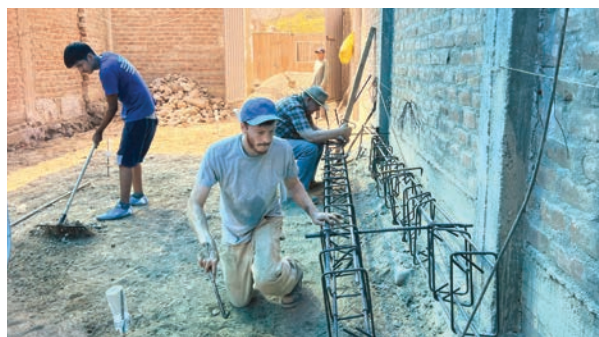
From top: Fred Scott, Jedidiah Lichty, Nadia Keyser, Dicky Amaya, Mario Painemal, Justin Wallace, and Elias Welch break up the old concrete floor; As Jedidiah packs up, Dicky surveys the completed project; Jedidiah and Fred prepare rebar pillars while a young man from the assembly removes debris. Below: Nadia Keyser and Becky Hulshizer work with first graders.
